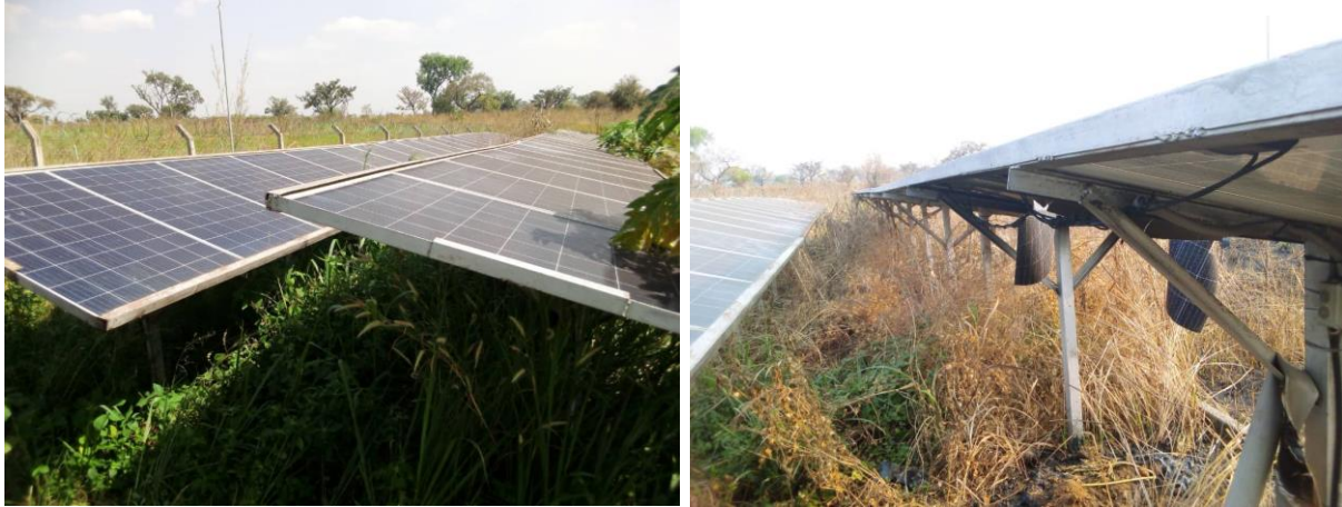
Figure 3 Aringo-Mone mini irrigation project; poorly maintained (Before and after photo) as documented by our Monitoring Officer Okot Churchill Peny-Can
